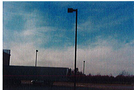
Exterior Lighting – Duplin Tech Center
