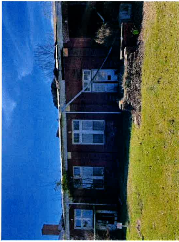
Sample were taken from the parapet wall and painting gray coating on the metal roof.
